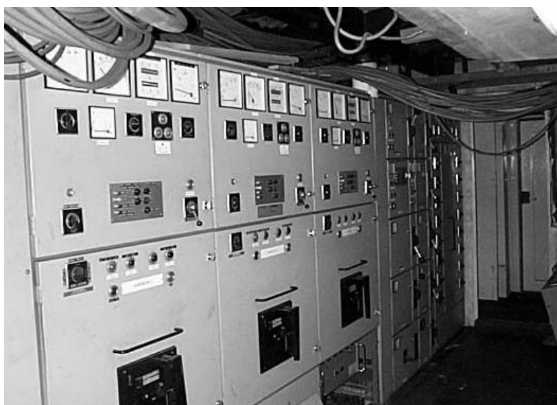
Figure 13 A main electrical switchboard in a machinery control room
